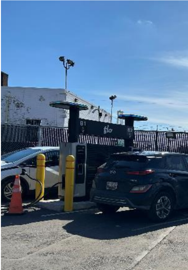
Benning Rd Fast Charger (4 ports) Ward 7 June 2025
