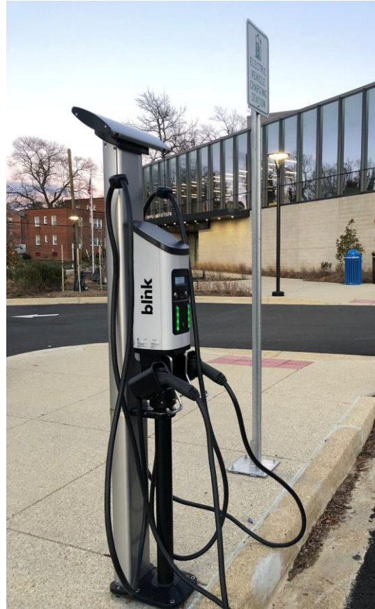
Fort Dupont Ice Arena Level 2 (5 ports) Ward 7 Dec 2025
